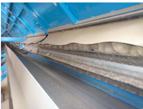
Driven out feed rollers, to secure even out-feed.
