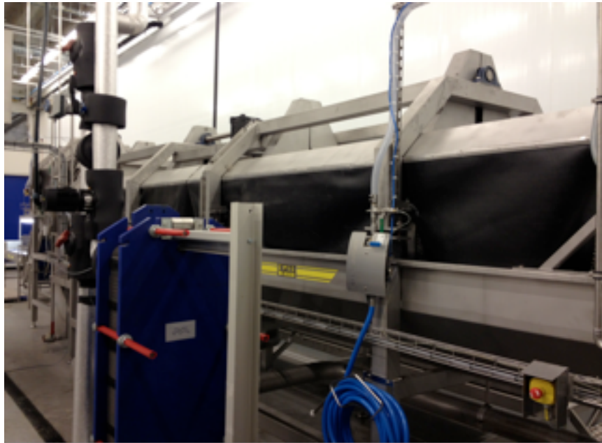
Machine with heat plate exchanger connected.
